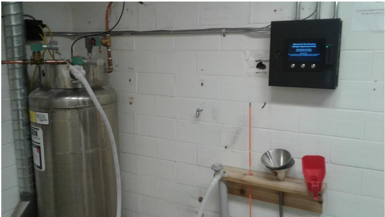
Figure 7 Open Dewar Filling Station
