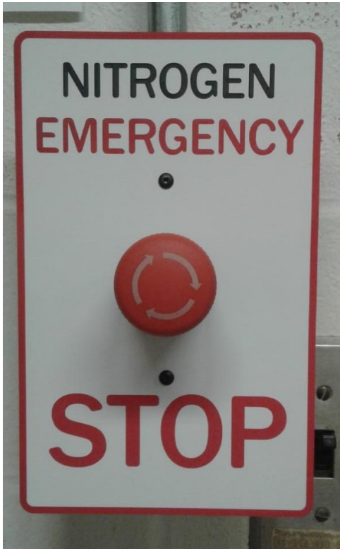
Figure 4. Emergency Stop button located beside main door.
